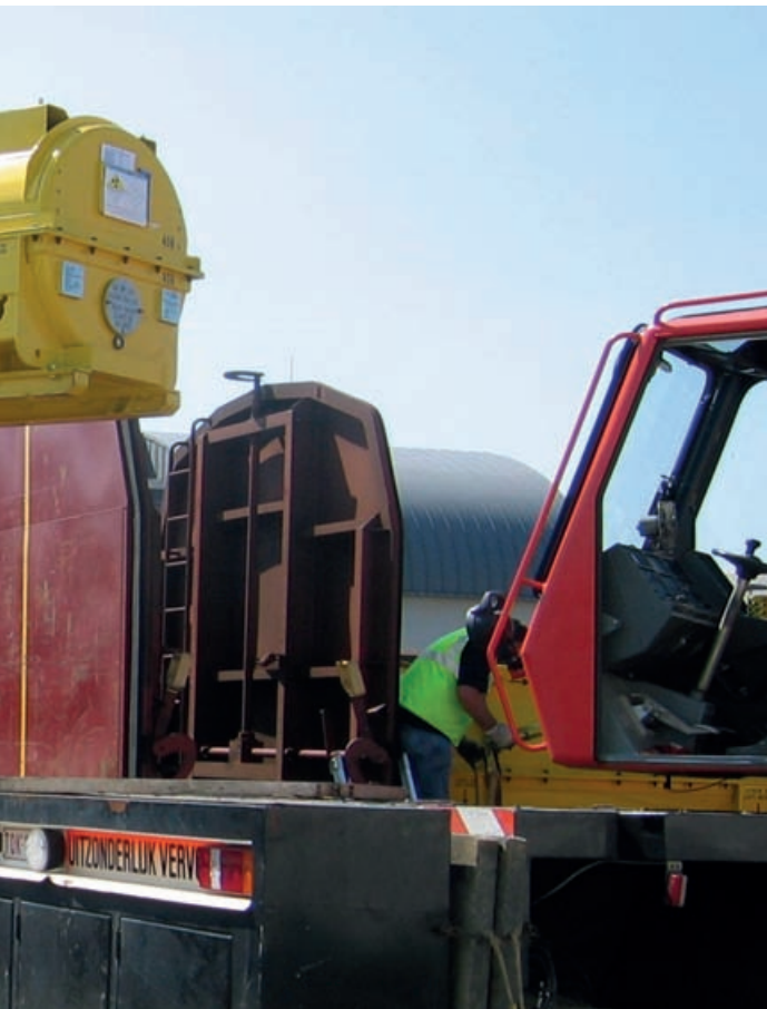
Loading a fresh fuel package onto a wagon
